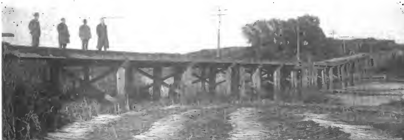
Free Bridge Over the Seneca River, Near Auburn, N. Y., Repaired by the Local Automobile Clubs
